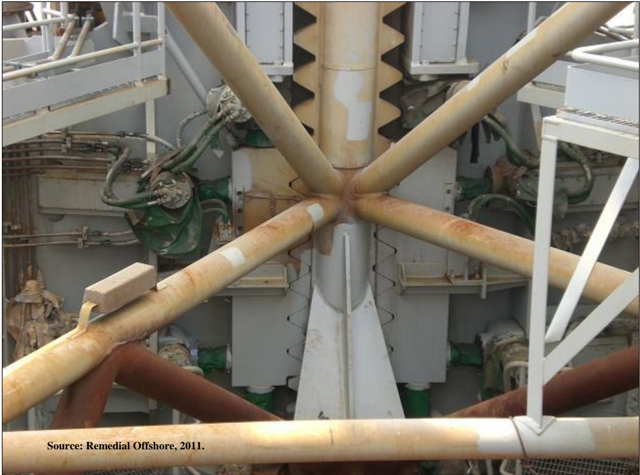
Figure H.8. Rack chocks are inserted against the leg's racks to transfer the vertical load away from the pinions.
