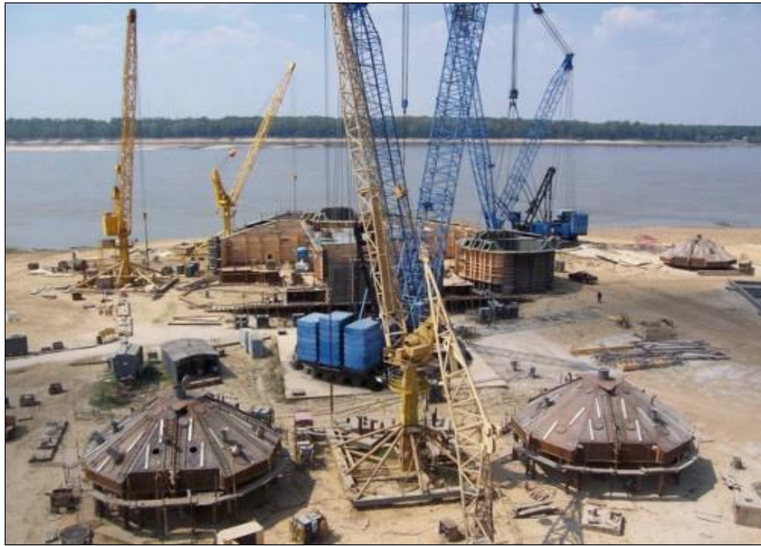
Figure I.2. Early construction stages of jackup rigs: F&G JU 2000E (top) and Hank Boswell (bottom) at the LeTourneau Vicksburg, Mississippi yard.
